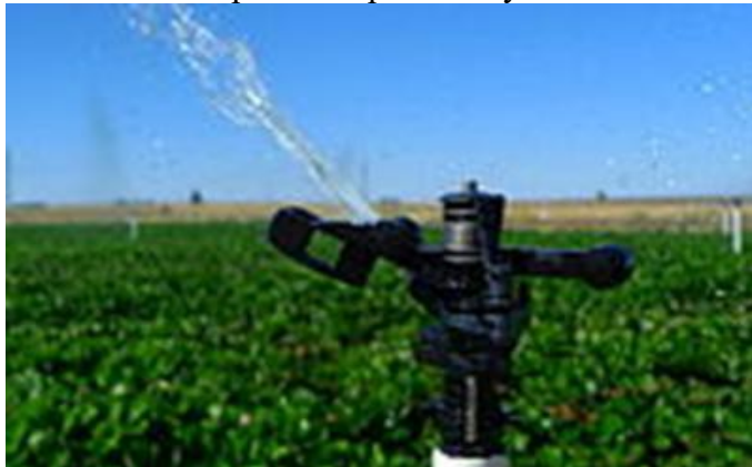
Sprinkler in operation
