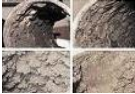
Fig.5.4: Scales Formed Due to Corrosion
