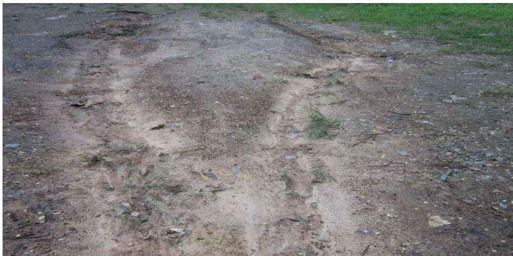
Fig. 3 Early stage of gully erosion
