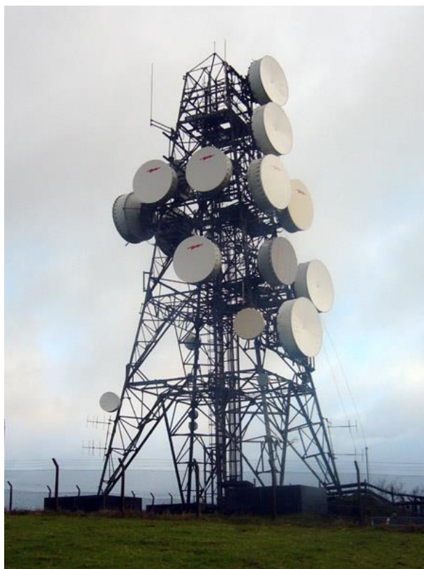
Figure 1.33: Microwave transmission station
